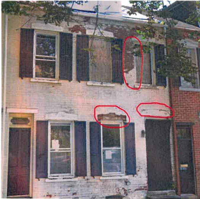
Front Elevation, Missing Window Header (Previous Application)
