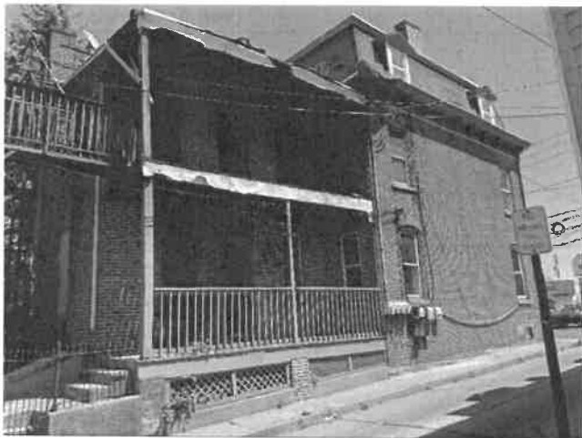
1021 Linden St after fire damage May 2023 (applicant)
