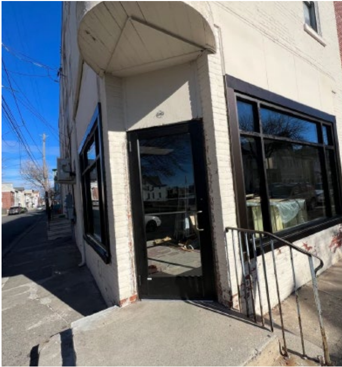
Aluminum entry door. (Applicant)
