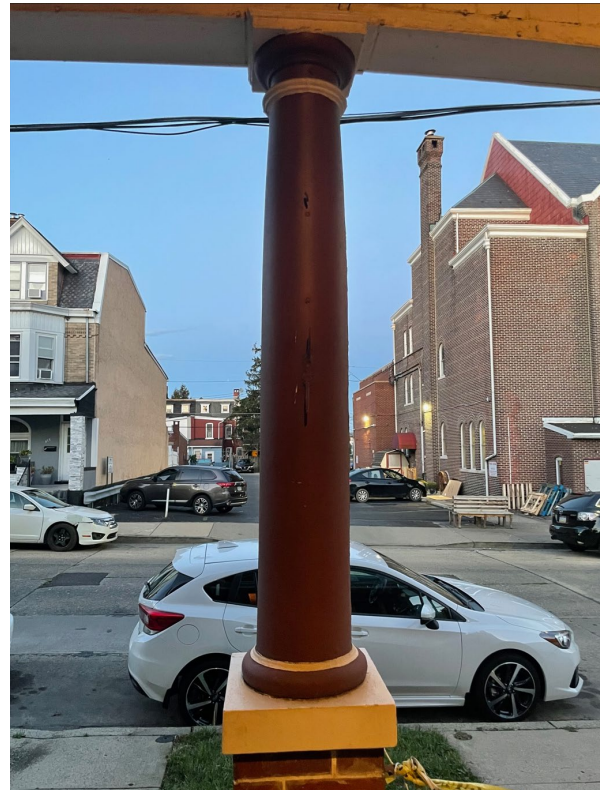
Porch column to be replaced, 2023. (Applicant)
