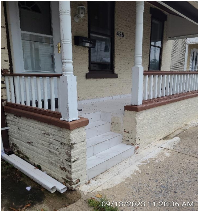
Photo showing the installation of tile on the front porch and steps of 425 N. 10th Street, 2023. (Staff Street View)
