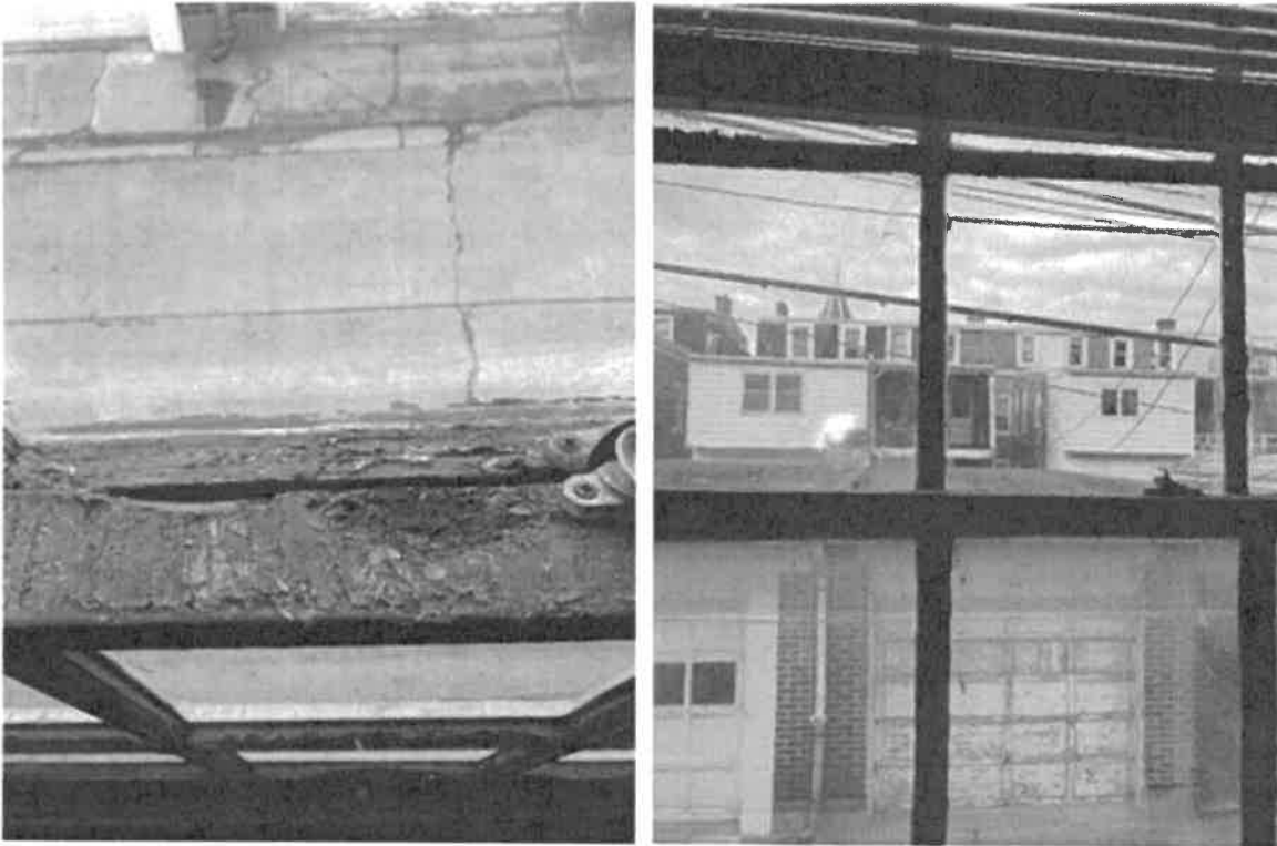
View: West side of the building in alley, first floor; window is damaged, doesn't work.
