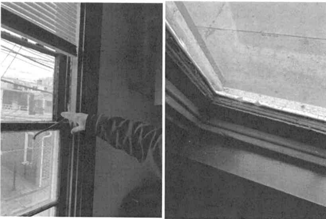
View: West side of building in alley, first floor; window doesn't work, gaps at the bottom, broken pulls.
