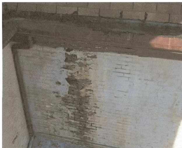
Damaged Wall Paint (Applicant)
