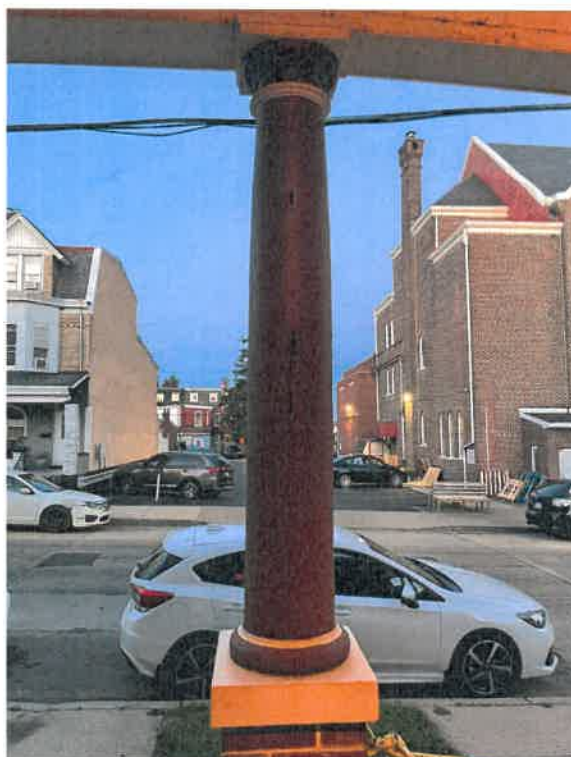
Porch column to be replaced, 2023. (Applicant)
