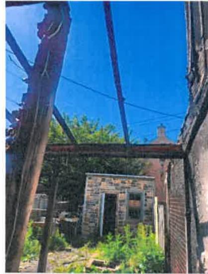
Fire Damage at Building Rear (Applicant)
