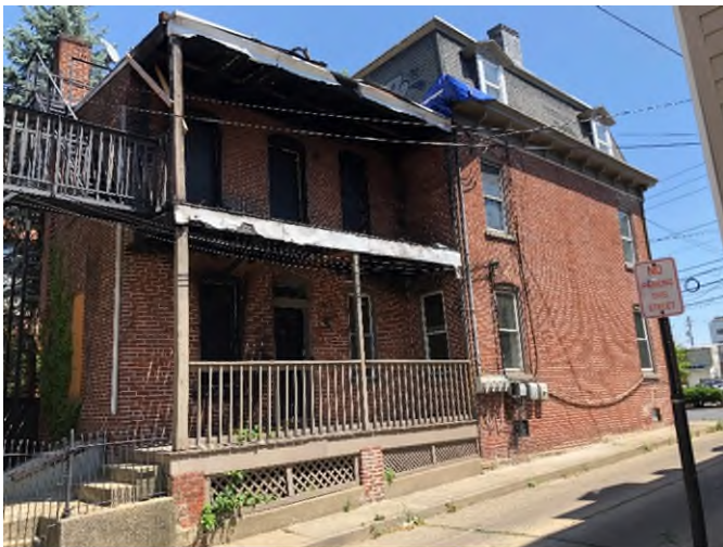
1021 Linden St after fire damage May 2023 (applicant)
