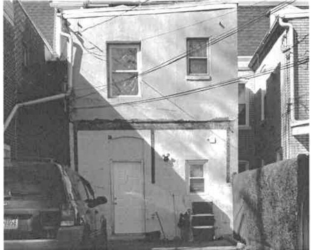
Rear of 141 N. 10 th Street following removal of the porch roof, 2023. (HARB files)
