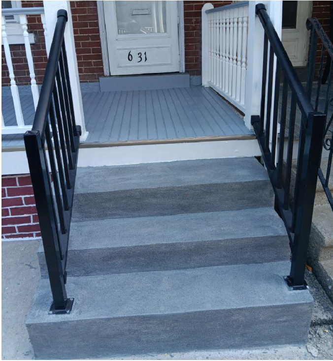
Steps and metal railings not reviewed by staff, 2023. (Applicant)
