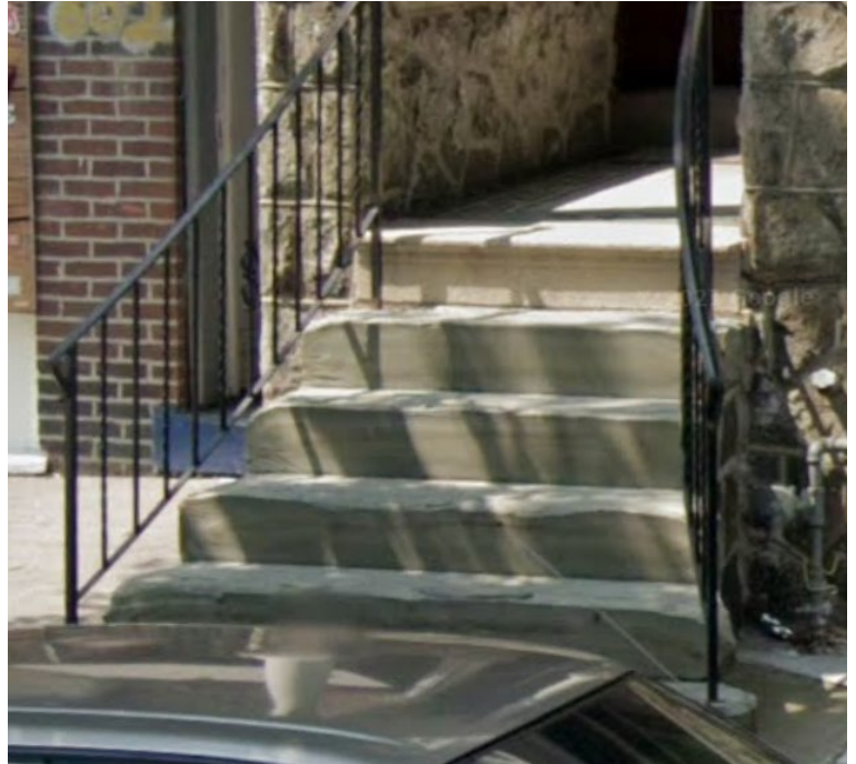
Detail of the stone steps prior to the concrete repair, 2021. (Google StreetView)
