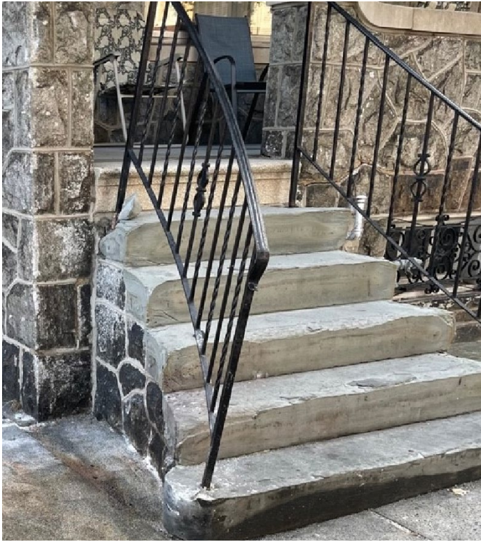
Photo showing the damage sustained following an accident before the coating was applied. (Applicant)
