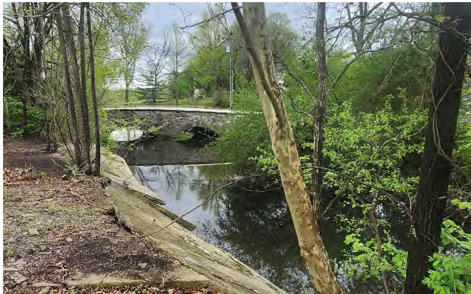
Dislodged, obsolete concrete slab embankment armoring threaten the historic Walnut St Bridge. City-partnership investments to solve these erosion/floodplain issues are essential to protect MLK Trail improvements to be installed directly downstream through Union Terrace Park.
