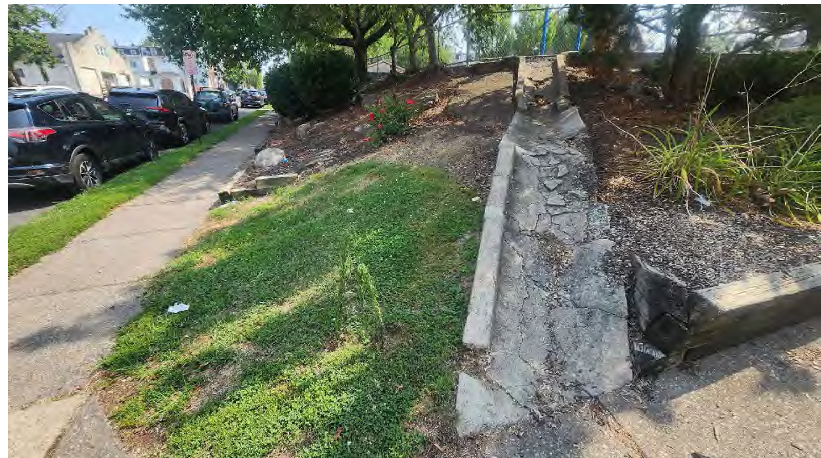
Stormwater is conveyed off of Franklin Park and into the streets by way of this deteriorated runnel system.
