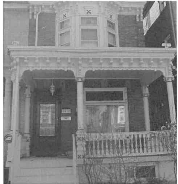
Original decorative wood porch balusters, railings, columns, and capitals, c. 2004. (HARB files)
