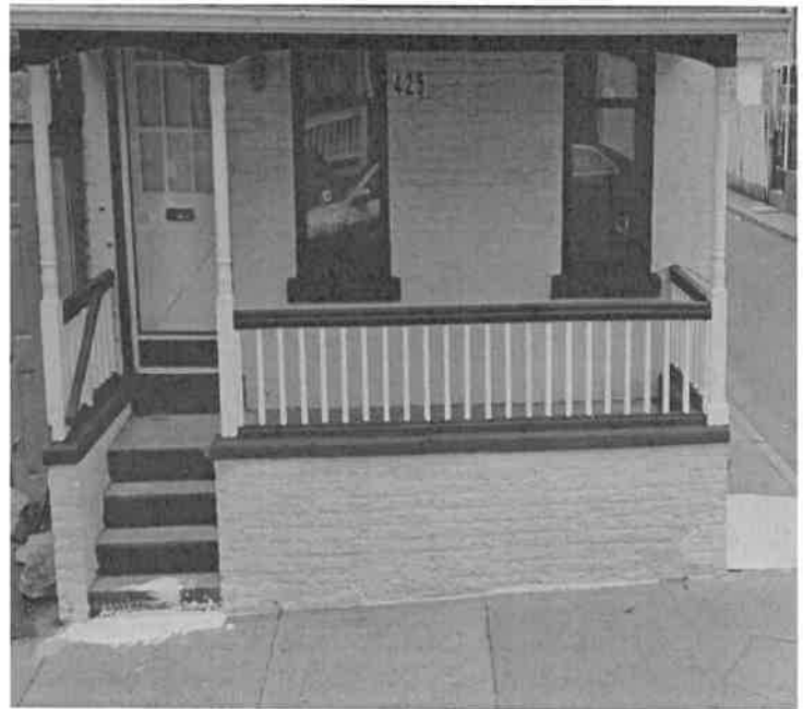
Photo showing the condition of the porch and steps prior to alterations, 2019. (Google Street View)
