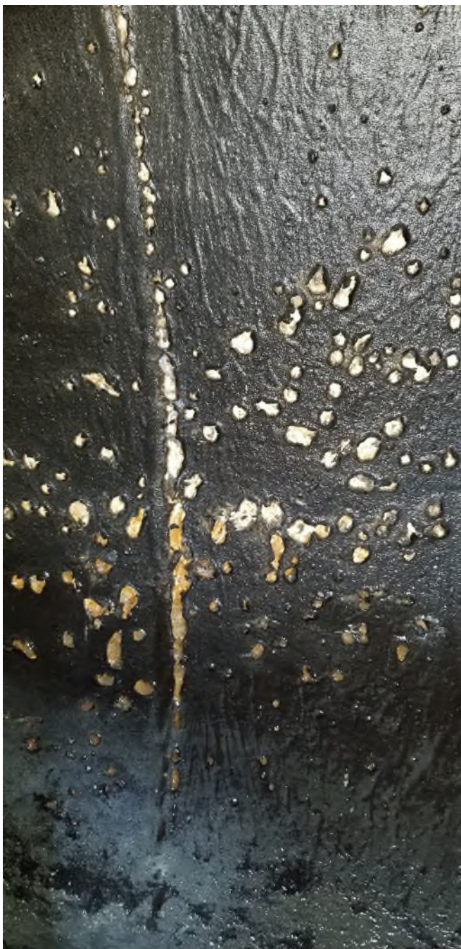
Figure 22 - ARV 6 toward ARV 5 - Coating Blisters and Disbondment
