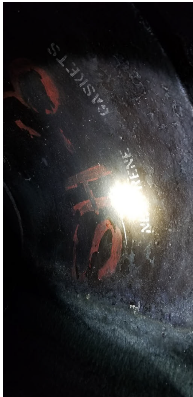
Figure 30 - ARV 9 - ARV 8 Pipe Wall
