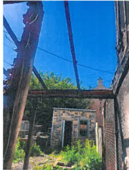
Fire Damage at Building Rear (Applicant)
