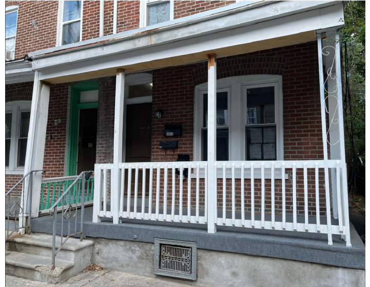
Rear of 141 N. 10 th Street following removal of the porch roof, 2023. (HARB files)
