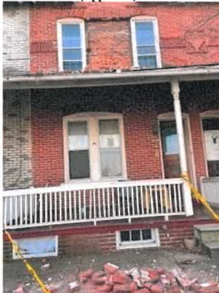
Damaged Primary Facade (Applicant)
