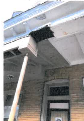
Existing Header (Applicant)
