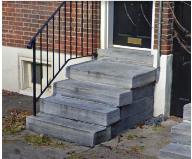
Image showing detailing with steps overhanging cheeks. (Google StreetView)
