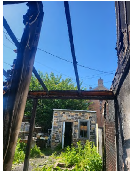
Fire Damage at Building Rear (Applicant)
