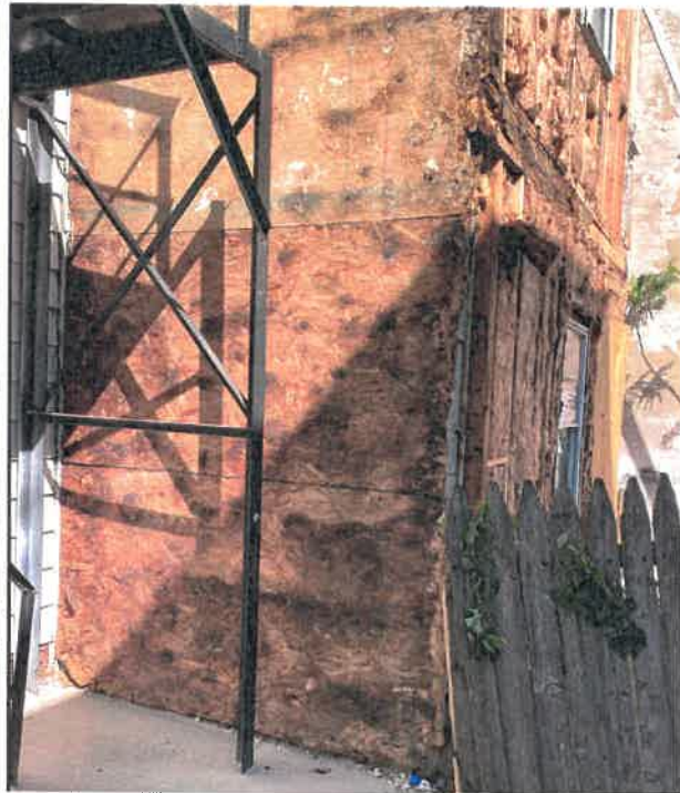
Photo showing the wall condition following stucco removal. (City of Allentown)
