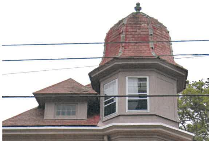
1550-52 W. Chew Street turret roof in 2019. (Google StreetView)
