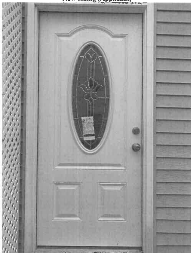
New Door Location (Applicant)
