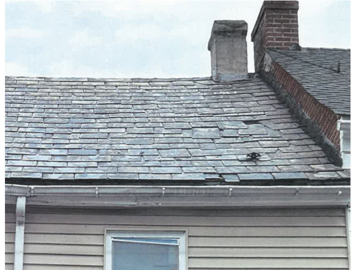
Condition of rear roof, 2023. (Applicant)
