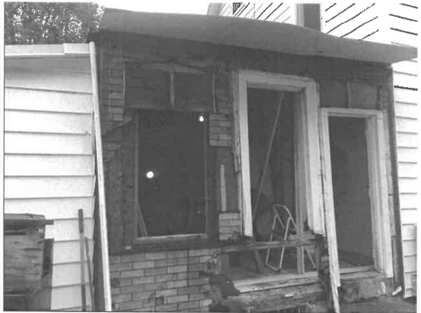
Photo of the rear ell following the removal of the siding. (HARB files)
